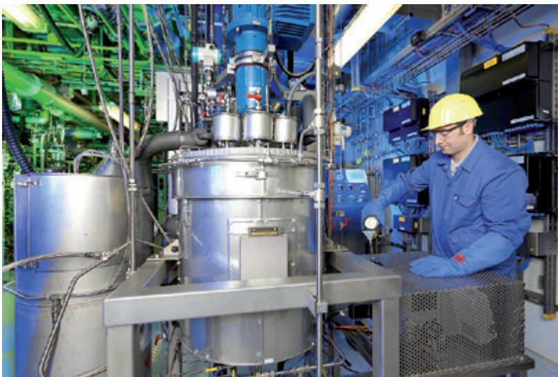
Fig. 6: Completed Mini Plant for the production of \text{CO}_2 -containing polyols
