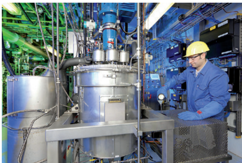
Fig. 16: The completed mini-plant for the production of CO 2 -containing polyols
